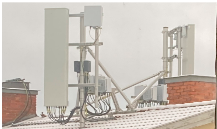
Figure 2: Picture of the 5G base station with antennas directed towards the studied apartment.
